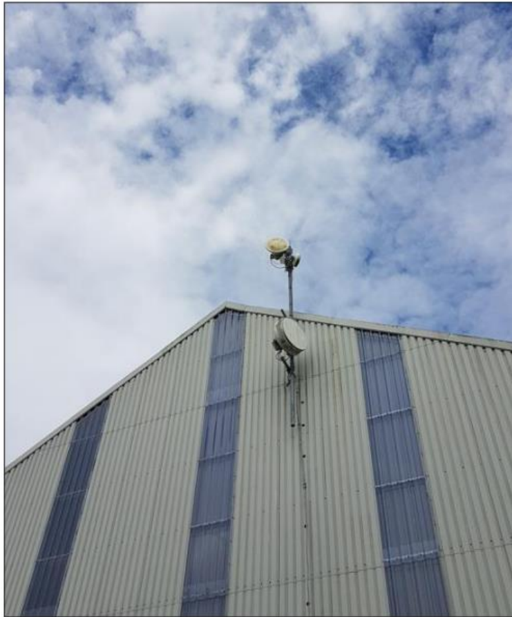
Fig. 3 – Decommissioned Vodafone equipment on site at Bord na Móna Derrygreenagh
